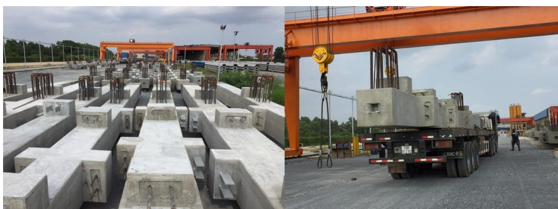
Figure 1. 8 Pipe Rack Column - the largest prefabricated precast concrete component in Viet Nam at Phan Vu Infrastructure Construction Co., Ltd
