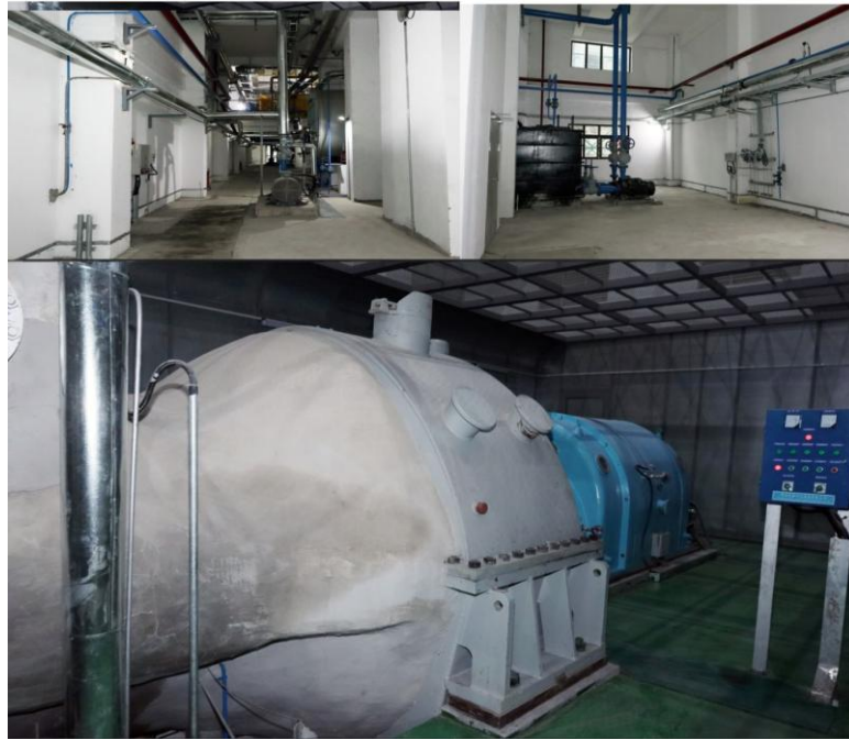
Figure 2. 13 WHR system at Vicem But Son plant (Source: Vicem But Son)
