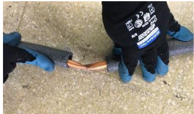
Figure 29: Inadequately handled copper tube (Source: HEAT GmbH)
