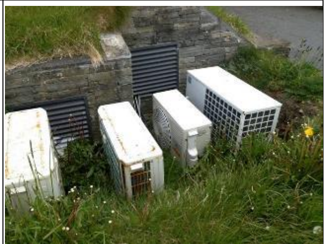
Figure 9: Example of inadequate outdoor unit installation (Source: HEAT GmbH)
