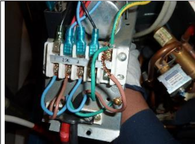
Figure 27: Example of inadequate electrical connections - no cable hoes or end splices (Source: HEAT GbmH)
